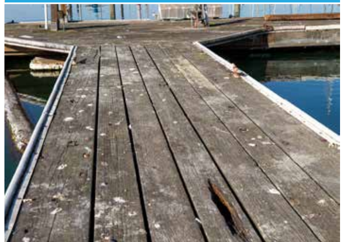
Deteriorated Marina Dock
